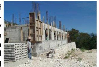
Village of Hope clinic under construction. Work on the 2nd floor has just begun.
